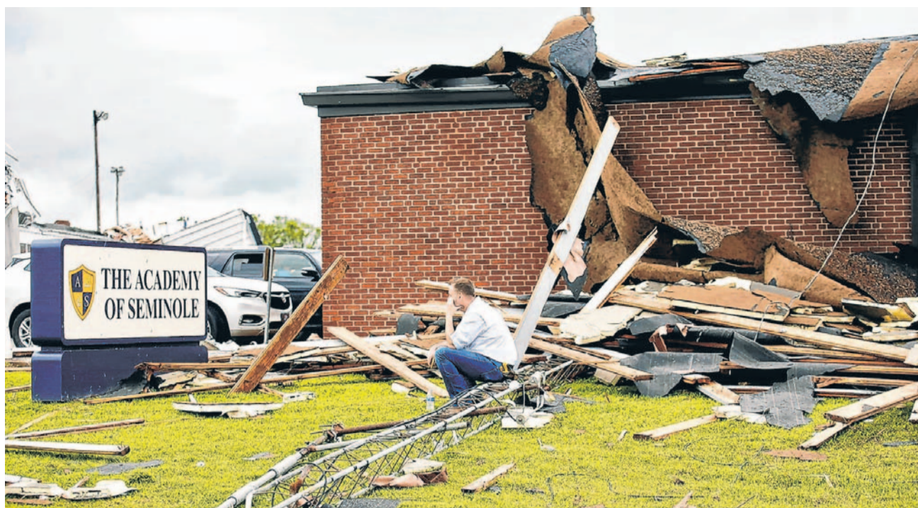
IN RUINS: Debris surrounded a school in Seminole, Okla., Thursday, the day after a springtime storm system spawned twisters that tore through areas of Texas and Oklahoma. Several structures were damaged but there were no reports of serious injuries.
