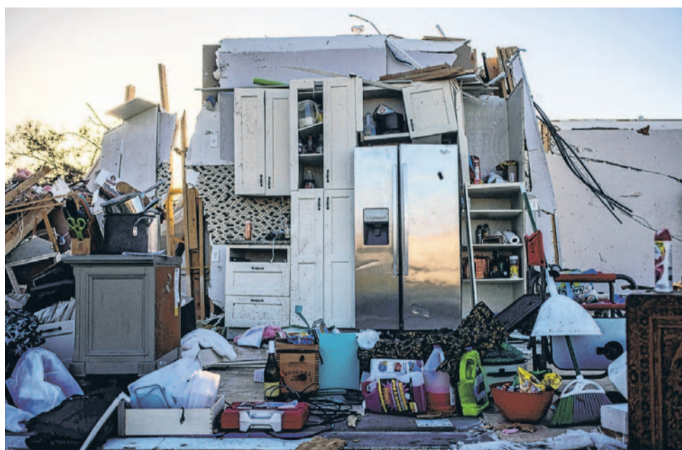
MAJOR LOSS: Part of a kitchen of a home left in ruins remained standing Thursday in the aftermath of a tornado this week that struck Arabi, in the New Orleans area.
