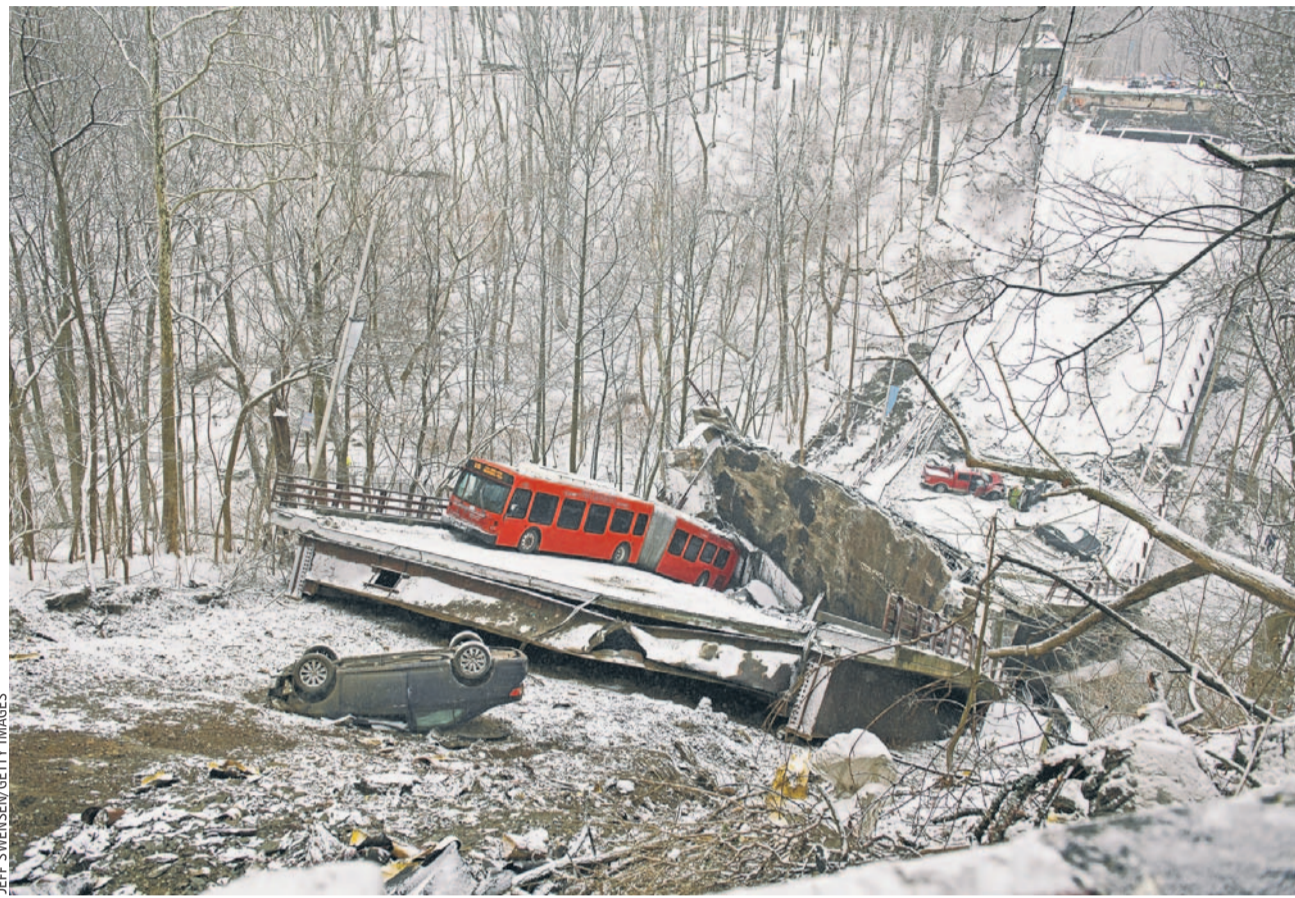
BREAKDOWN: President Biden stressed the need to invest in U.S. infrastructure on Friday as a planned visit to Pittsburgh coincided with the buckling of the span. Ten people were injured and a major roadway was disrupted. A4
